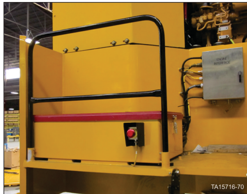
Figure 3: Battery box –side view
